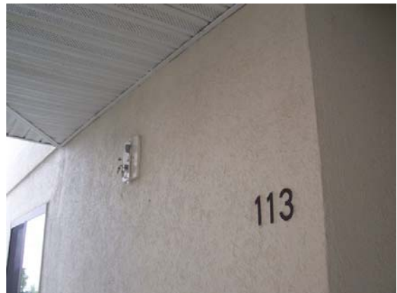
Photo 4 - Fire alarm and missing exit sign
