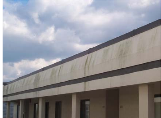
Photo 2 – EIFS system showing staining
