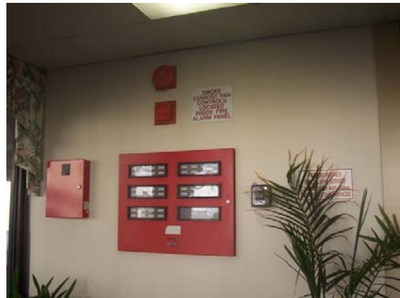
Photo 4 - Fire Alarm System
