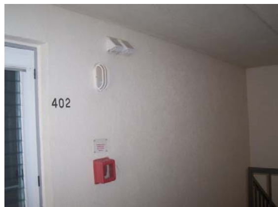
Photo 4 - Fire alarm and lighting system
