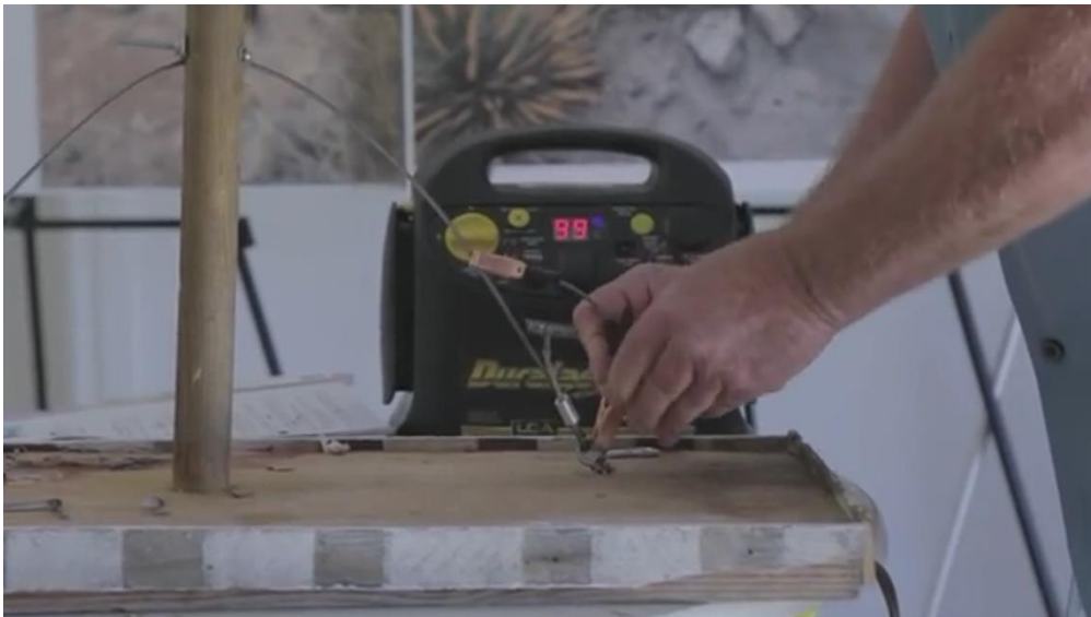
Photo 13 Shunt applied to down-guy and ground rod. Photo by Ed Clark
