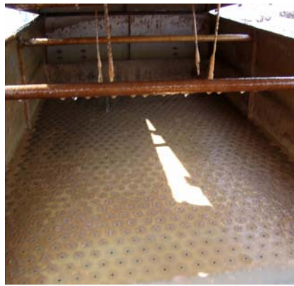
Fe Oxide/Hydroxide Fouling of Tray Air Stripper
