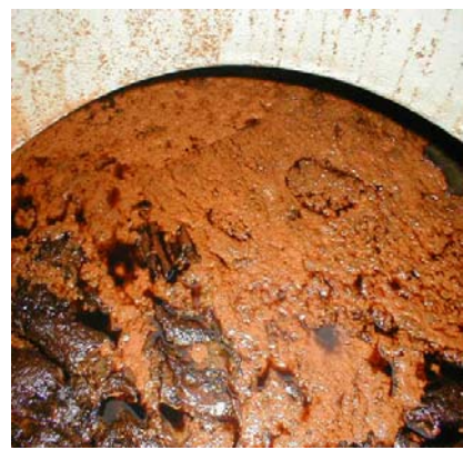
Biofouling of Oil-Water- Separator
