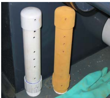
Inorganic Fouling (Iron) of Air Sparger
