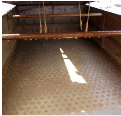
Fe Oxide/Hydroxide Fouling of Tray Air Stripper
